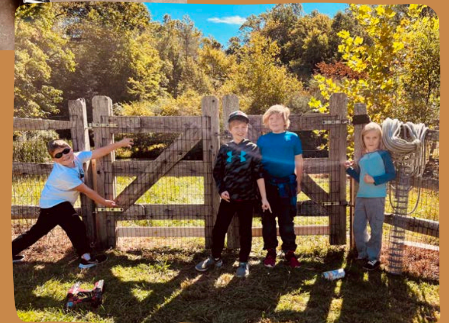
Jett, Josh, Wally, and Ollie are pleased with the fence repairs that Group I made so that the goats won't sneak through the fence.
